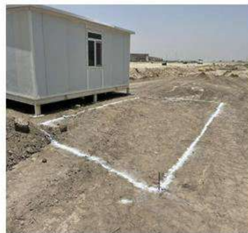
b. Photo for test room.
