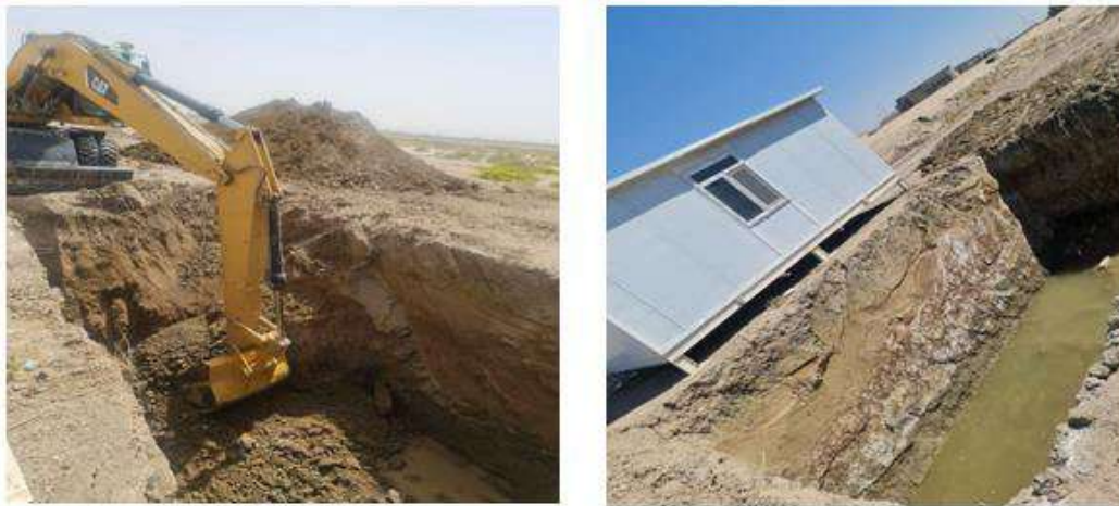
c. Excavation work. d. Hall. Fig. (1): Work of excavation in the ground at depth of 3.5 m.
