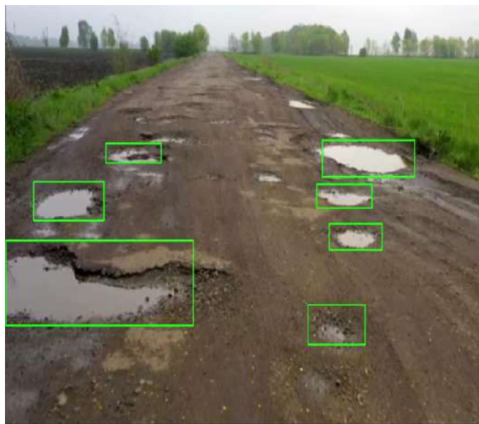
Fig 7 Potholes detected using YOLOv4 tiny
