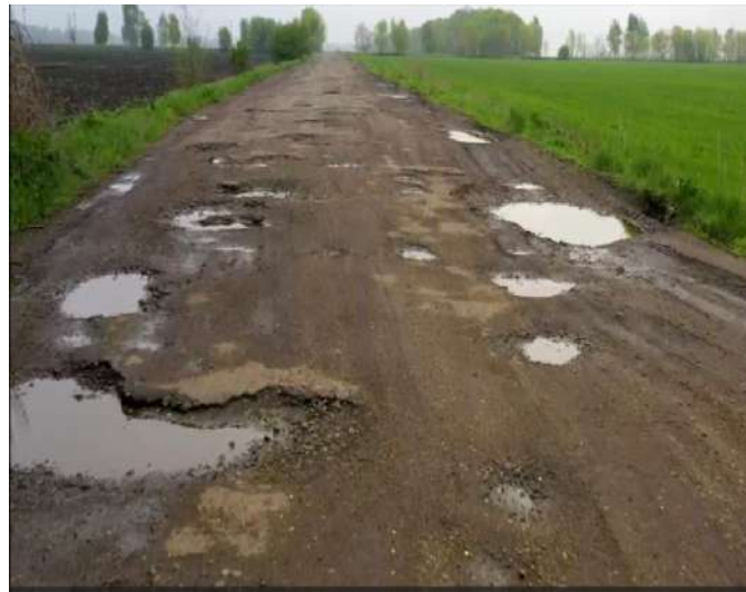
Fig 6 Potholes on road
