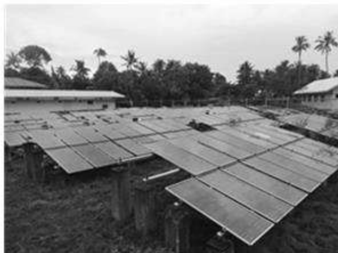
Figure 3. Condition of the Solar Panels of the PV System
