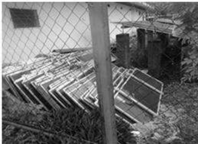
Figure 5. Defective panels of Pangan-an Solar Plant
