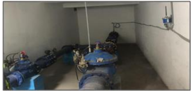
Figure 4 Integration Of The NEMOS N210 Datalogger With The Pressure Reducing Chamber
