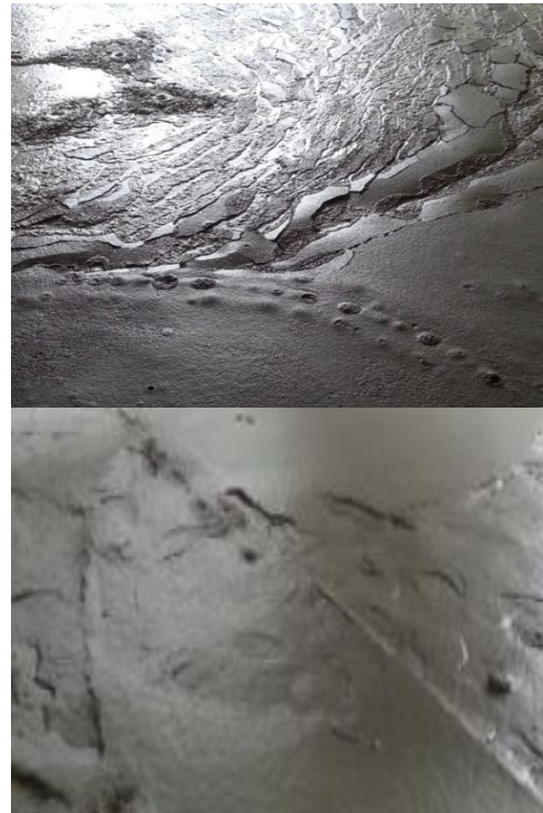
Fig. 3: Settlement and crack of CLC
