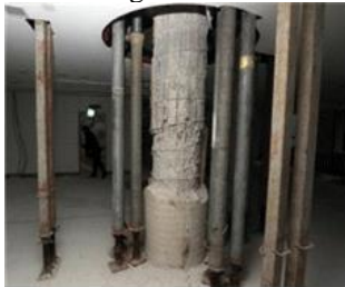
Fig 1: Column collapse in site
